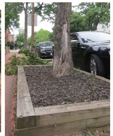
This planting box restricts free flow of rainwater, raises the soil level and creates a tripping hazard
